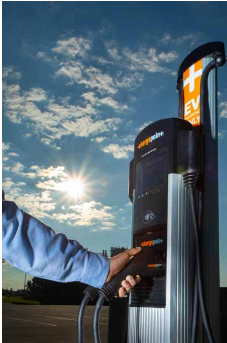
Batteries of two electric vehicles can be charged simultaneously at the new charging station in the Cajun Field parking lot.
